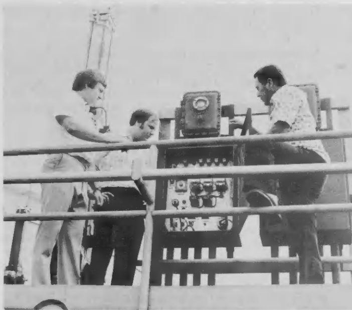
Tom Paddrik, Ben Kalis and Angel Rasmijn checking a pump control panel.
